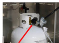
Regulator connected to propane tank
